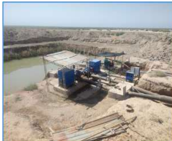
Water pumps in Jayhun district
